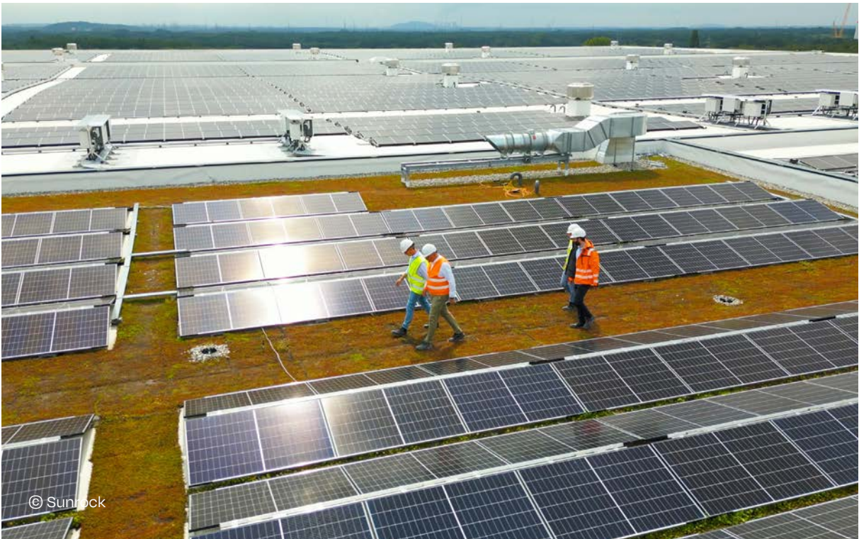
3.45 MW solar plant, Dorsten, Germany
