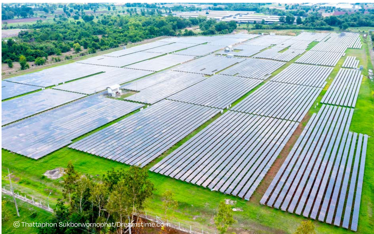
Solar power plant in Thailand
