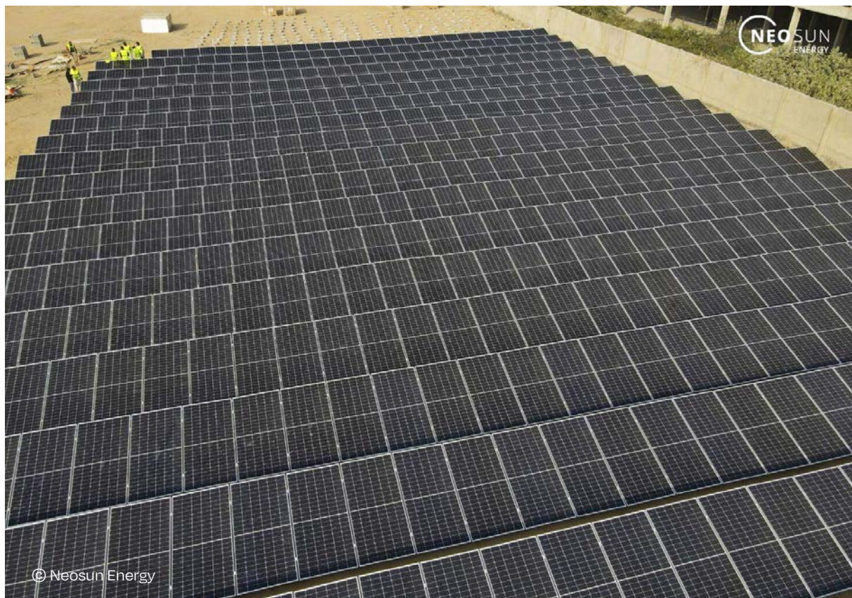
1 MW solar plant (phase 1 of 2 MW total) for Unity Foods Ltd, Pakistan
