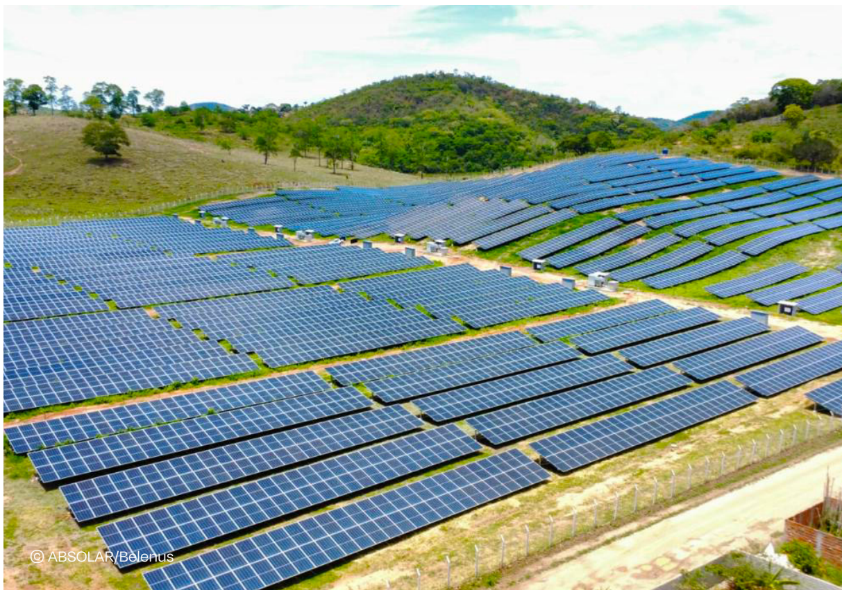
5 MW UFV Poté solar PV plant, North of Minas Gerais, Brazil
