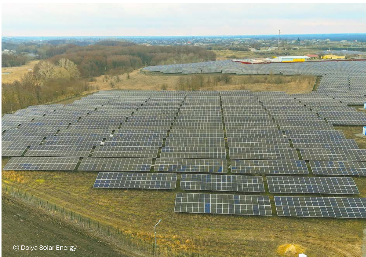
5 MW solar plant, Cherkasy, Ukraine
