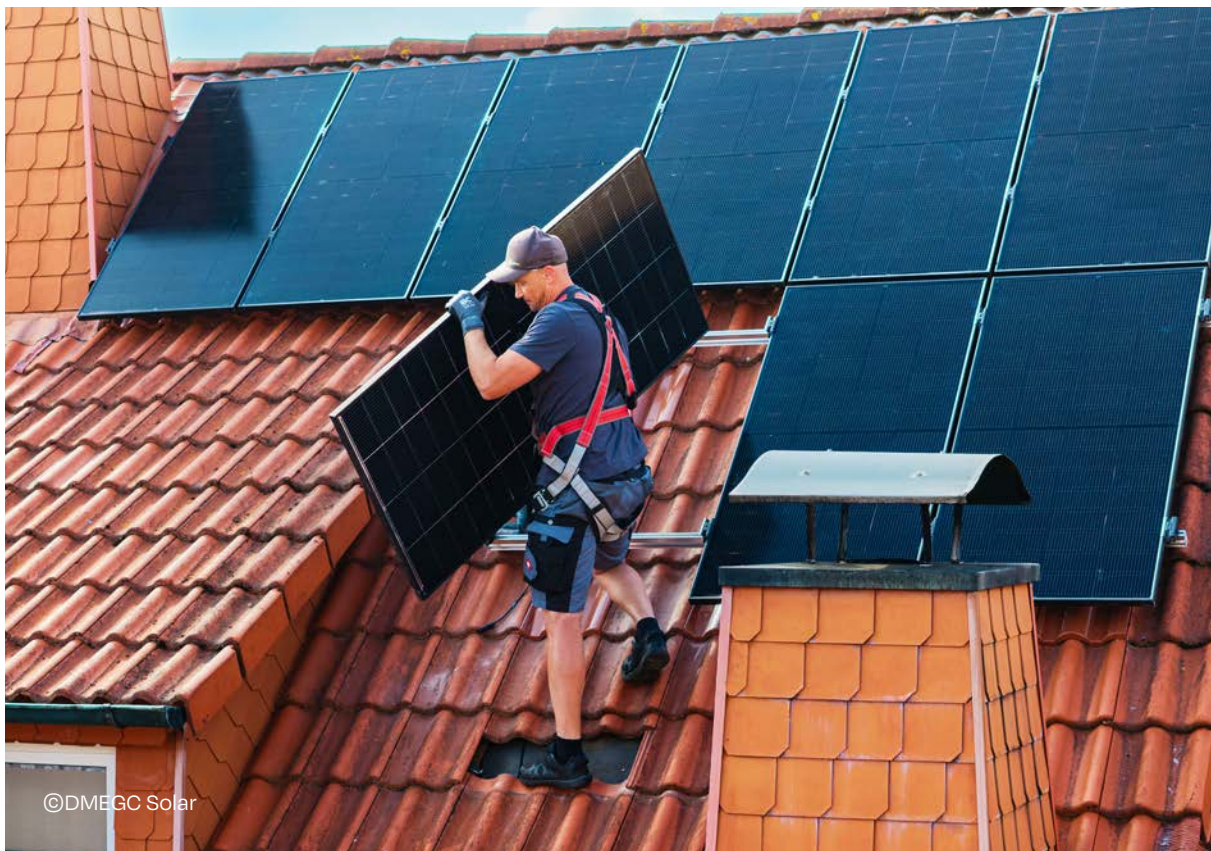
6.9 kWp rooftop solar installation, Germany
