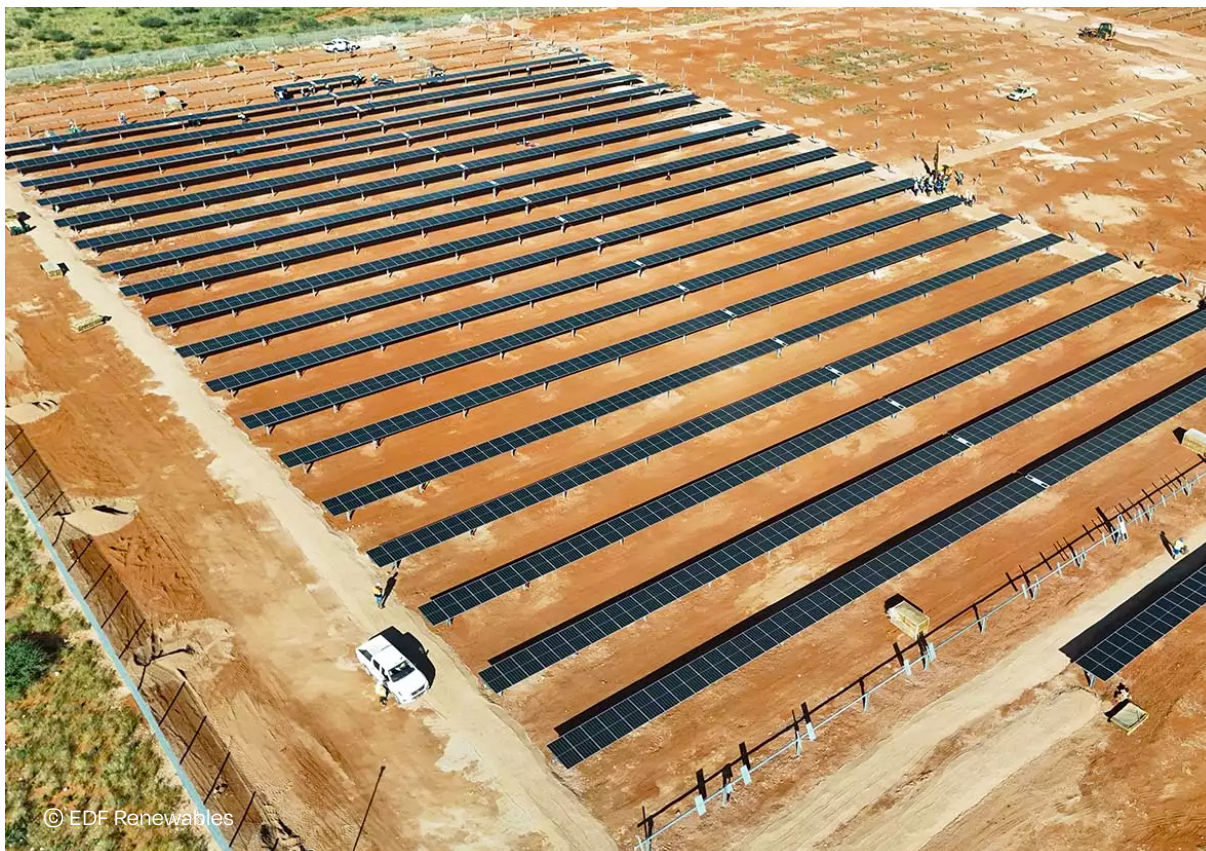
115 MW solar PV and 90 MWh BESS Umoyilanga Hybrid Project (RMI4P), South Africa
