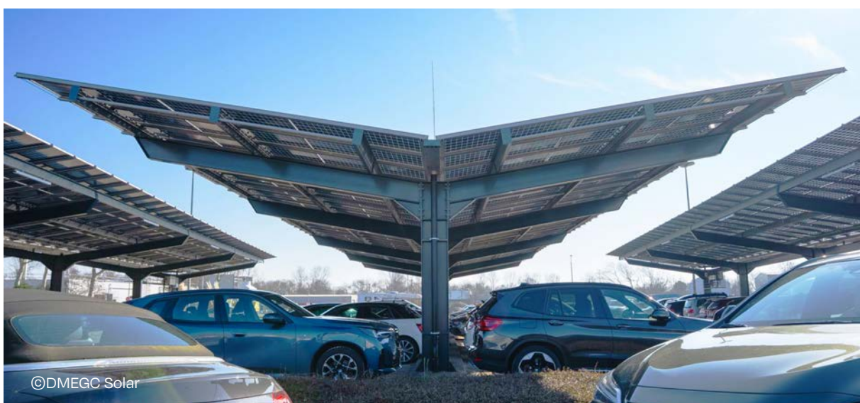
574 kWp solar carports, The Netherlands
