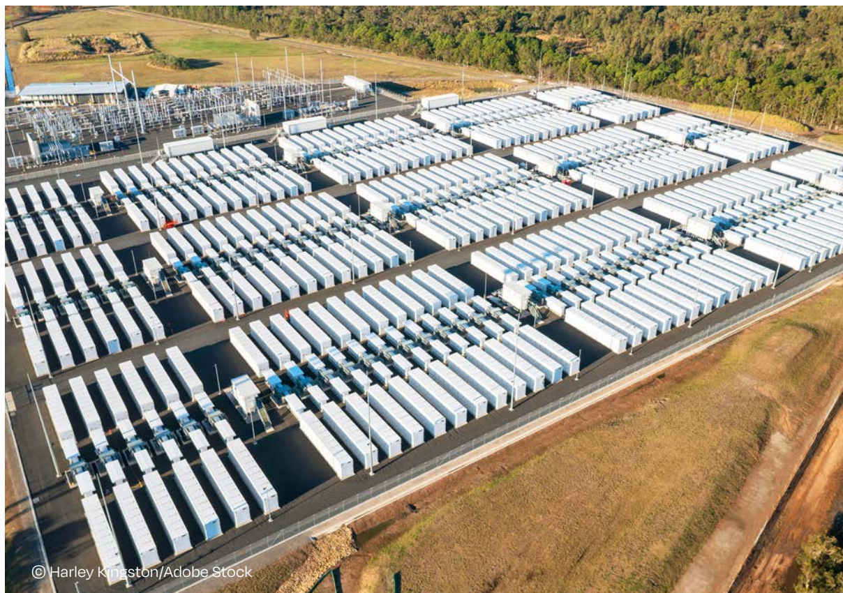
Waratah Super Battery at Colongra, NSW, Australia. Completed in 2025, 850 MWh battery energy storage system
